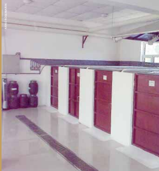
The urban onsite organic fertiliser plant at our project in China produces 1.5 tonnes of fertiliser a day from human manure.
